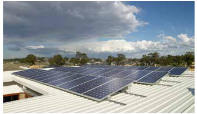
Solar Panels: Solar photovoltaic panels on the north side of the roof
