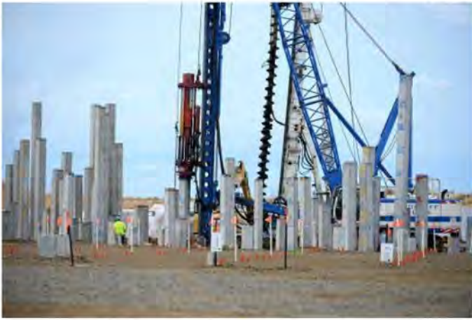
UNDER CONSTRUCTION: A skeleton of the Knauf plasterboard factory is beginning to take shape at Bundaberg Port.
