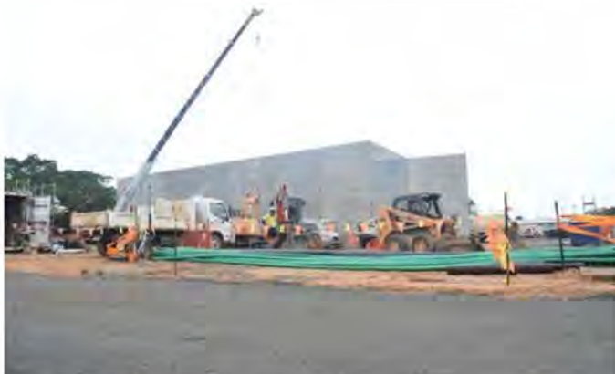
UNDER CONSTRUCTION: The first stage of the multiplex, a $14.5m sports centre, under construction on Kensington St.
